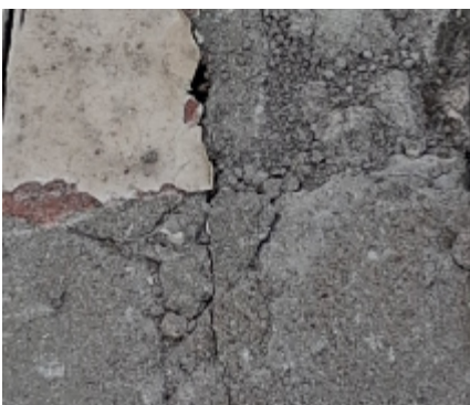
Fractured concrete substrate
